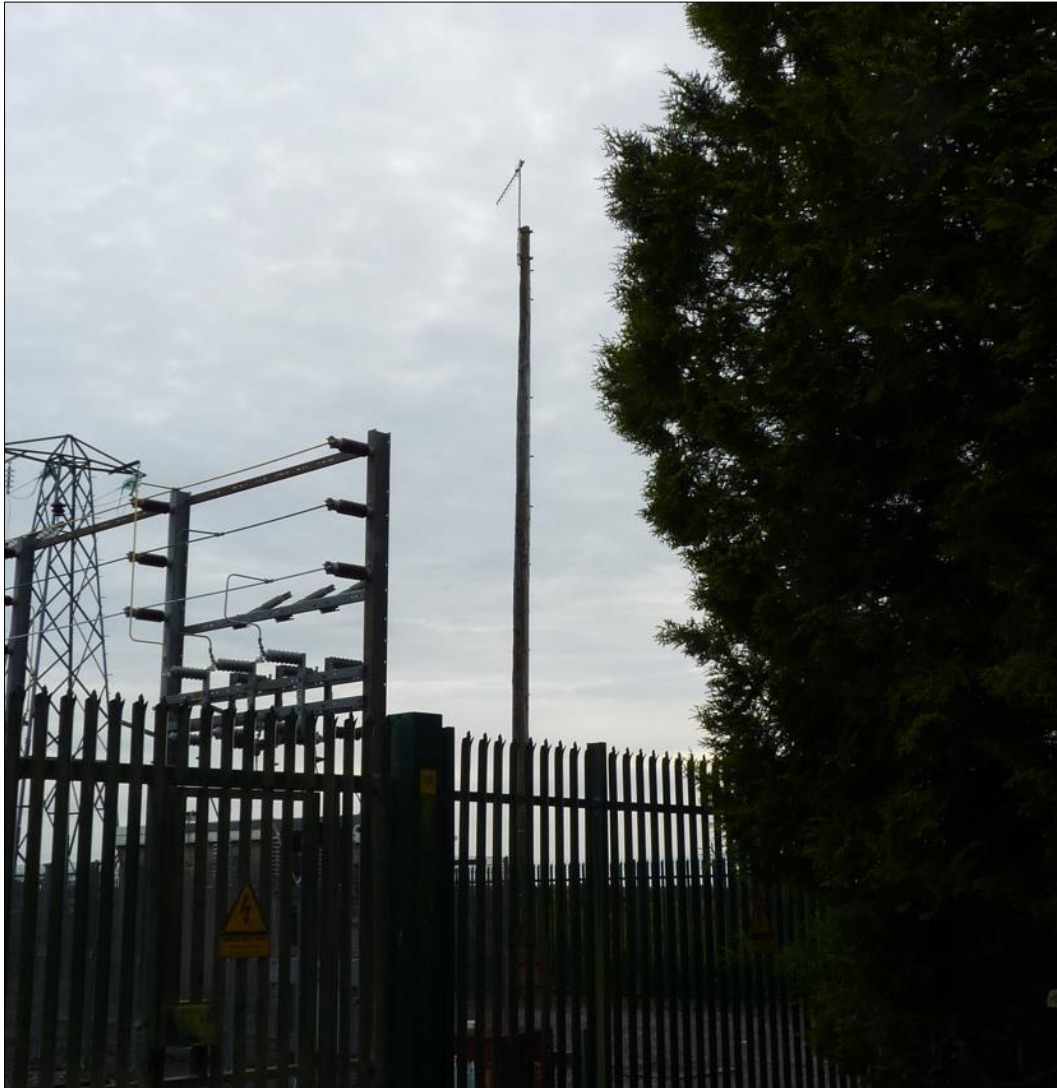
Figure 4. ESB Antenna at Glenamaddy 38kV Station
