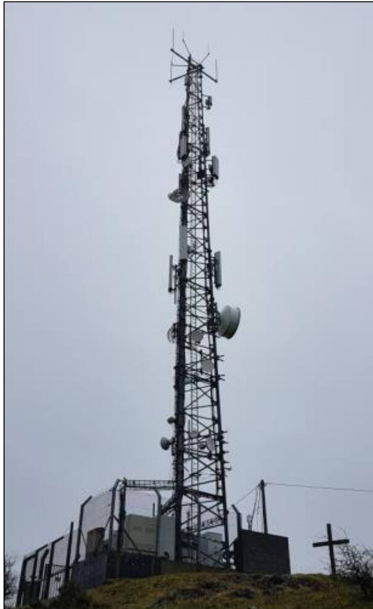
Figure 3. ESB Antenna at Abbeyknockmoy Telecoms Mast Site
